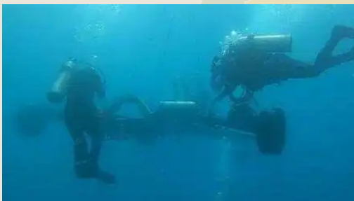
INDIA: A 2,300 kms submarine optical fibre cable network inaugurated by PM Modi in Andaman and Nicobar Islands. Credit: Hindustan Times
